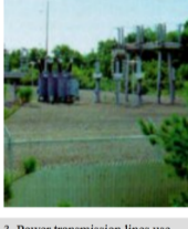
3. Power transmission lines use zinc-nickel coatings on anchors, cleats and bolts that connect lines and components.
